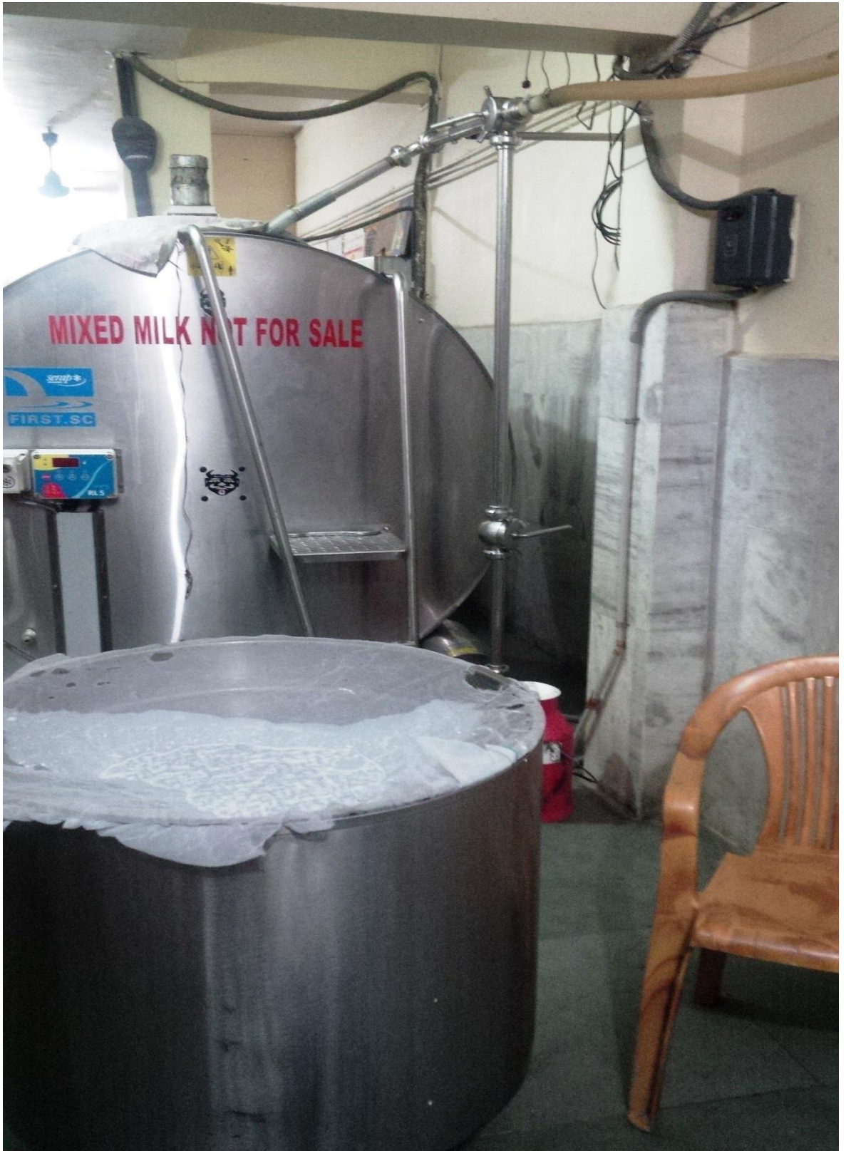
Photo 4.2 Bulk Milk Cooler (BMC) installed at VCS
